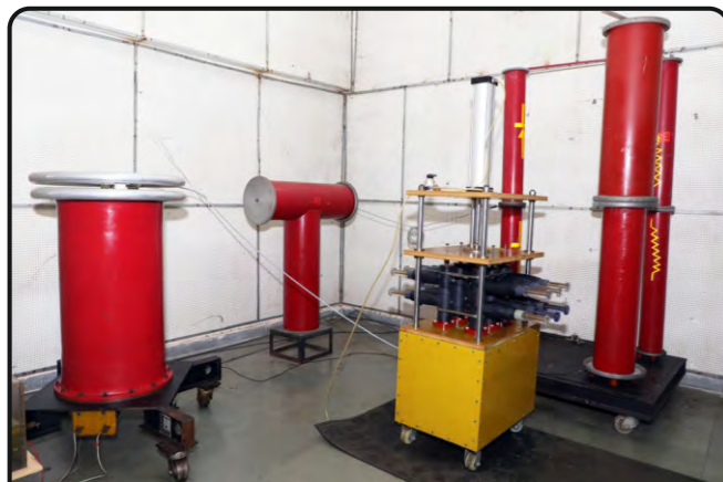
High Voltage Test Lab
